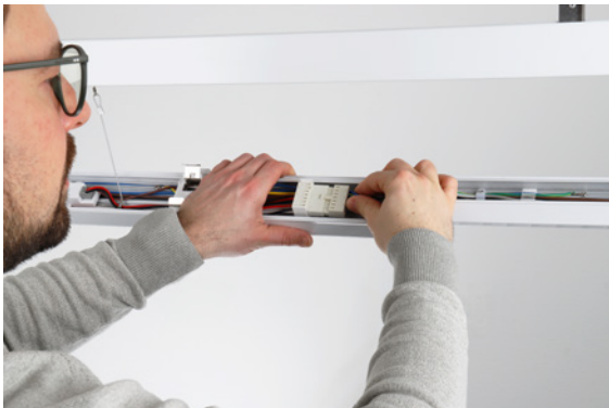
3 - connect modules and adjust power if necessary
